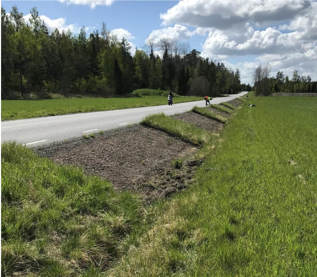
Figure 7.8: Over a number of years, a layer of more or less nutrient-rich organic topsoil builds up on the nutrient-poor road construction material. Competitive species become more and more dominant, and the topsoil layer compromises the drainage of the road. If the vegetation is still rich in species of conservation concern, patches of vegetation can be saved when scraping off the top layer, as dispersal cores for re-establishment of species. Knivsta, Province of Uppland, Sweden 2020.
