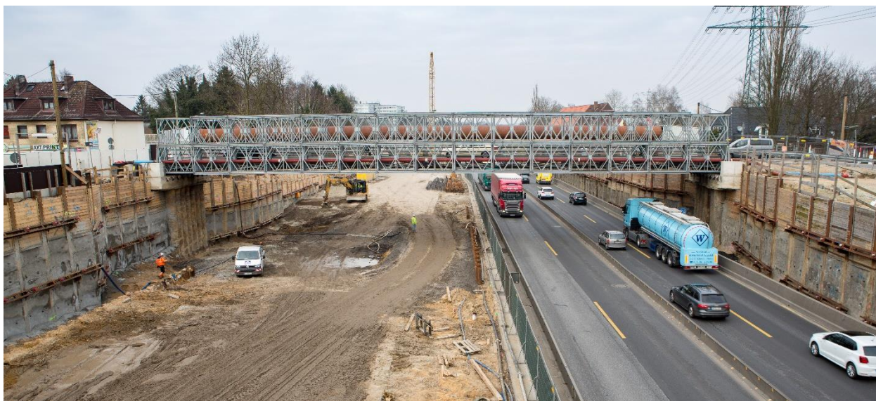
Figure 22: Situation during construction phase – traffic shifted to one side and reduced speed limits are introduced.
