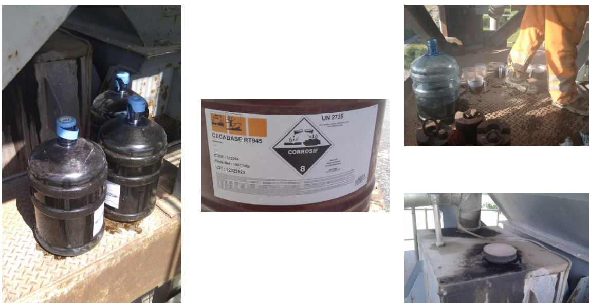
Figure 4-3: The warm mix additive and plant access point for dosing the mixtures
